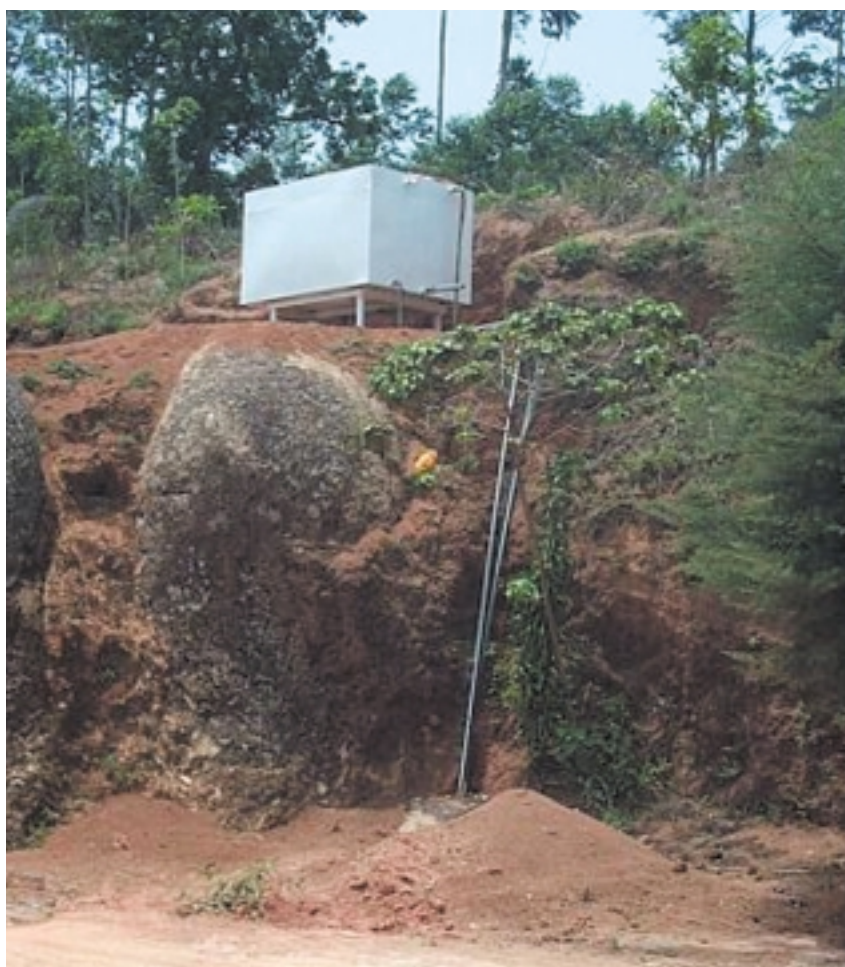
Figure 2. The 4,000 litre drinking water reservoir, painted white to minimise heating of the water by the sun. The pump is turned on once or twice a week to fill the reservoir. When the reservoir is full the pump shuts off automatically. This system decreases the frequency with which the pump will operate, thereby increasing its longevity and avoiding the problem posed by the previous system. The pump should last between five and seven years, when it will need to be replaced. The electricity is paid for by the state and as monies are collected from patients and other users, over time there should be enough money for a replacement pump.
