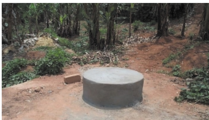
Figure 1. The completed well. It is sealed off with plaster to prevent contamination and people from easily removing the lid and tampering with the system. The pipe (now buried) extends from the well to the top right corner of the photo, toward the health centre.
